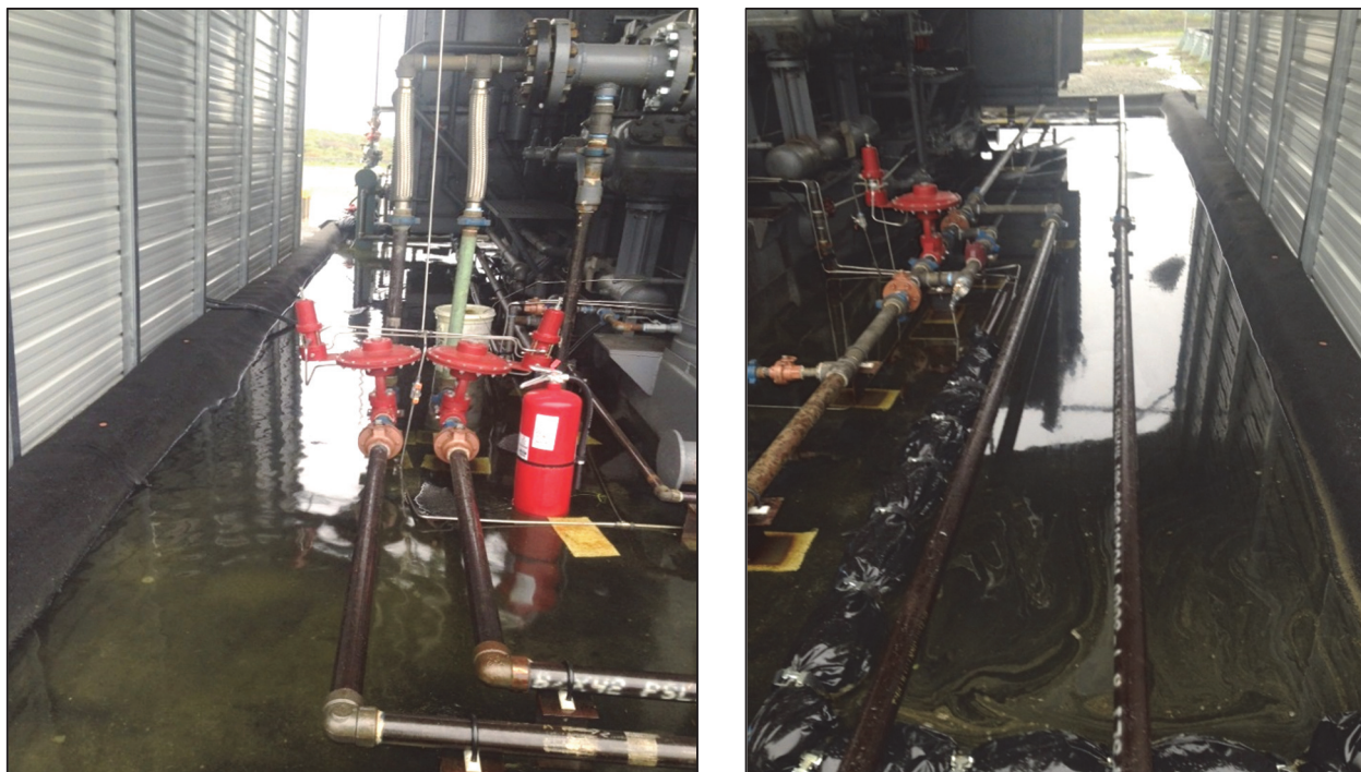
Figure 12: The concrete curb around this compressor package trapped oil and rain water, causing an injury when an operator tripped over a hidden obstacle and fell.
