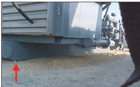
Figure 13: The end of this compressor skid is not well supported.
