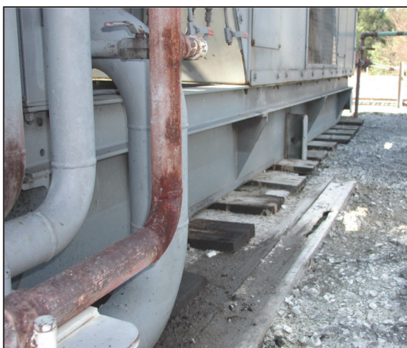
Figure 16: Non-permanent (e.g., rental) package on a swamp base foundation.
