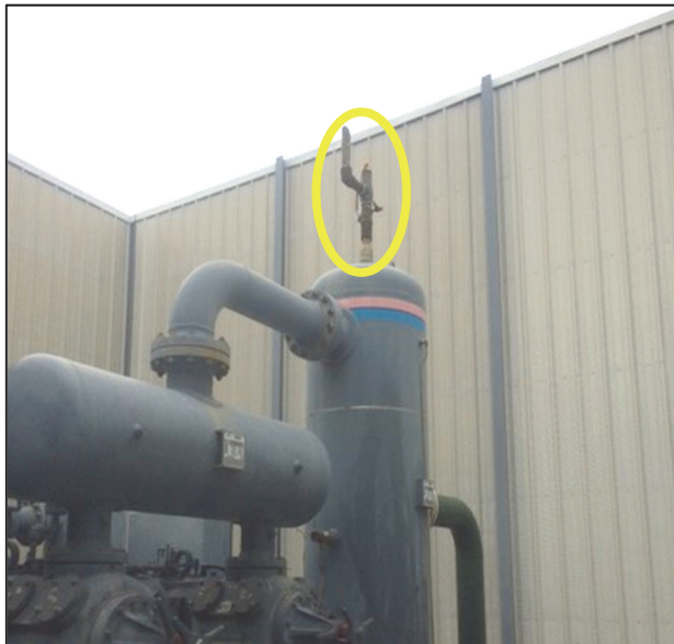
Figure 7: A small PSV mounted on top of a suction scrubber.
