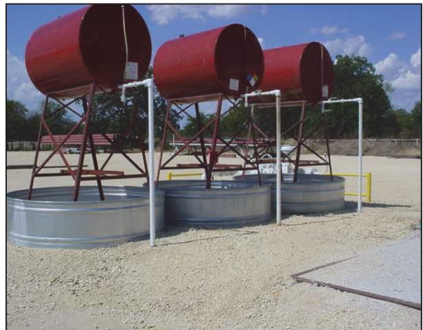
Figure 6: Example of oil supply pipes run subsurface to skid, avoiding tripping hazards.
