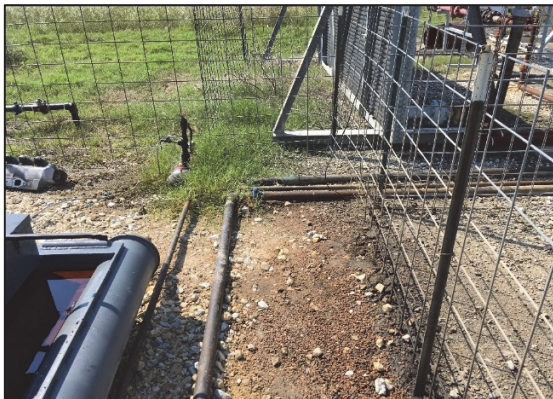
Figure 3: Example of an unsafe surface piping installation with trip hazards.
