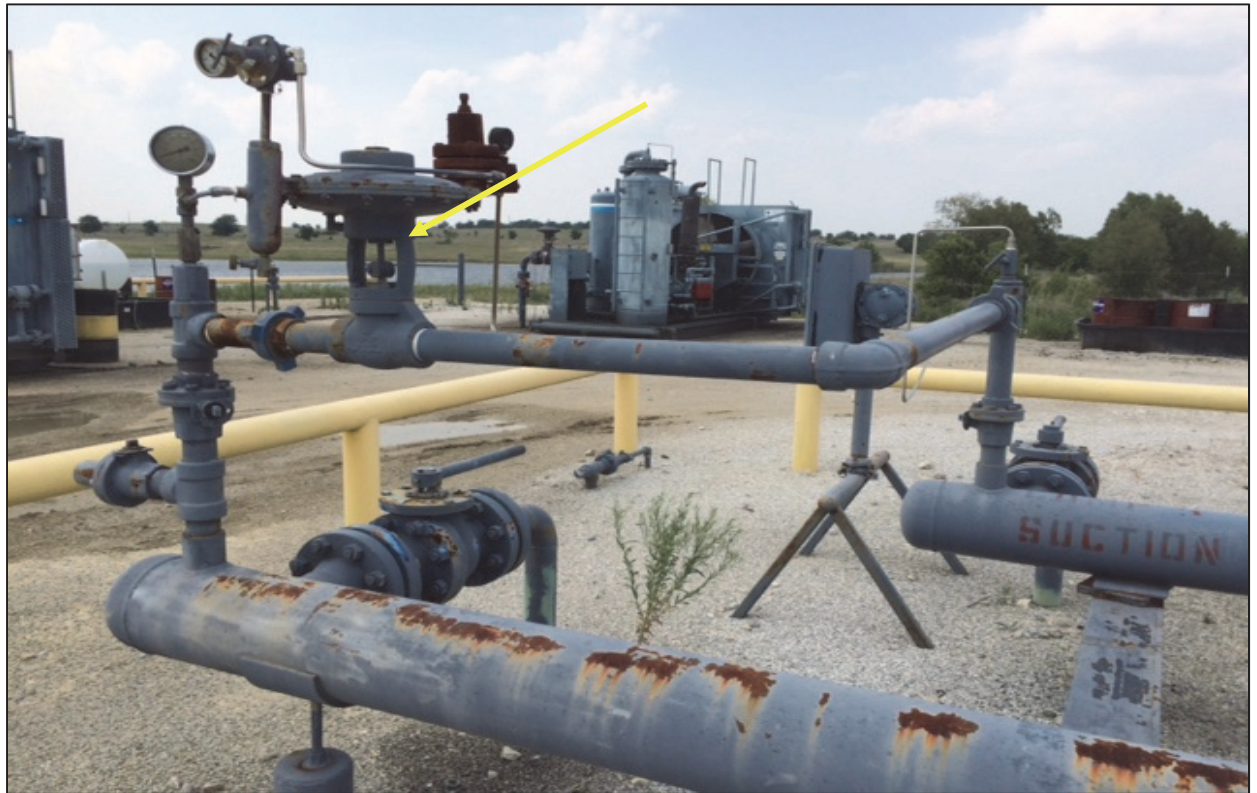
Figure 31: Connection of discharge and suction headers with an automatic valves to provide a recycle system for two screw compressor packages at a booster station.
