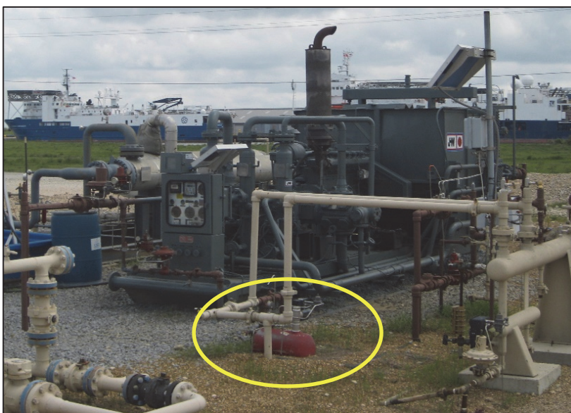
Figure 34: Blow case equipment captures fluids from the compressor skid and transfers them to a larger tank for disposal.
