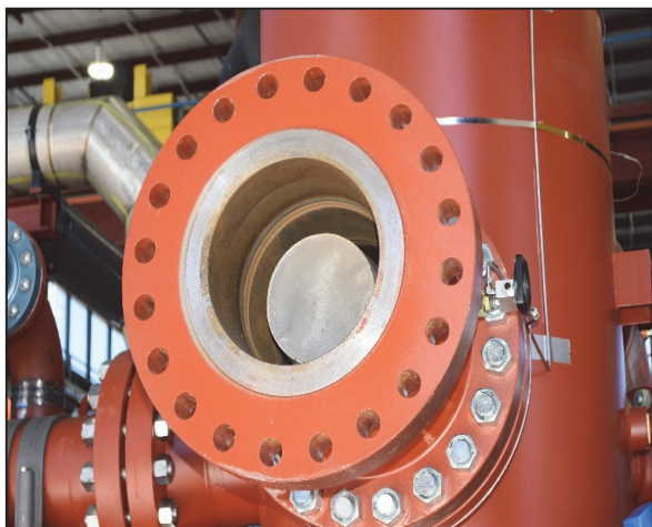
Figure 24: A debris basket strainer installed in a suction scrubber inlet.
