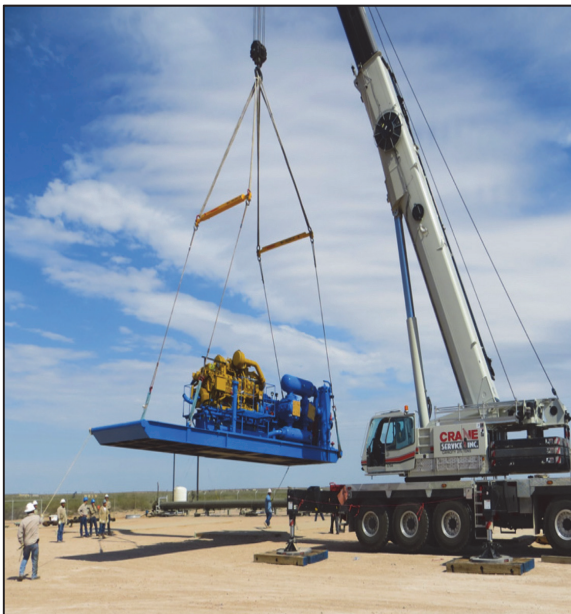
Figure 22: Larger horsepower packages are generally too heavy for a single lift.
