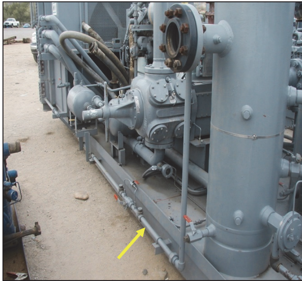
Figure 28: Starting bypass line designed into the compressor package.
