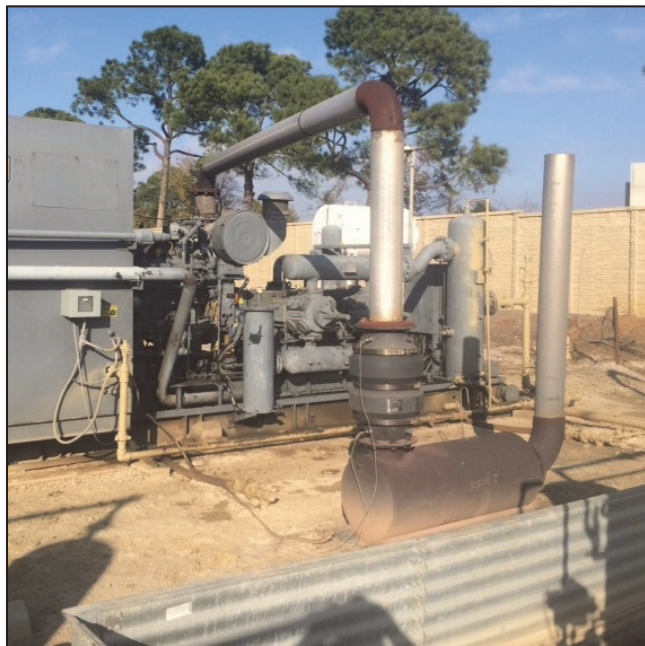
Figure 17: An exhaust silencer at ground level reduces sound travel over walls at an urban golf course. Insulation or a personnel barrier is missing.
