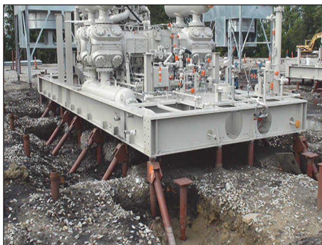
Figure 15: Compressor package and off-skid horizontal coolers both mounted on screw piles.
