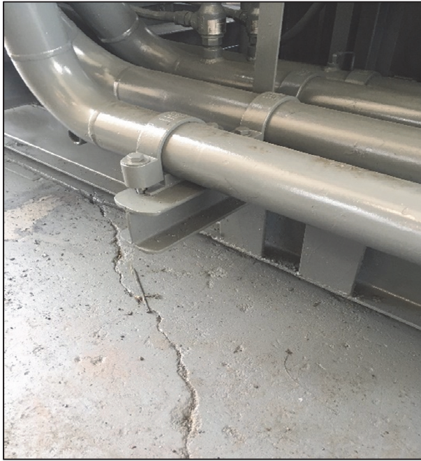
Figure 26: Use I-beams and pipe clamps to support piping. Note round corners for safety.
