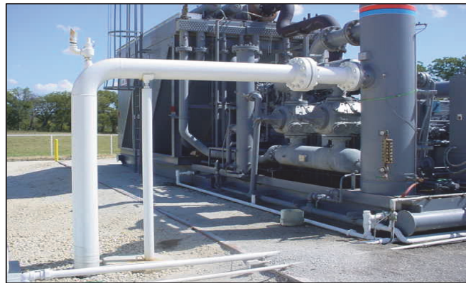
Figure 4: Example of a much better installation that allows a clear path around the package.
