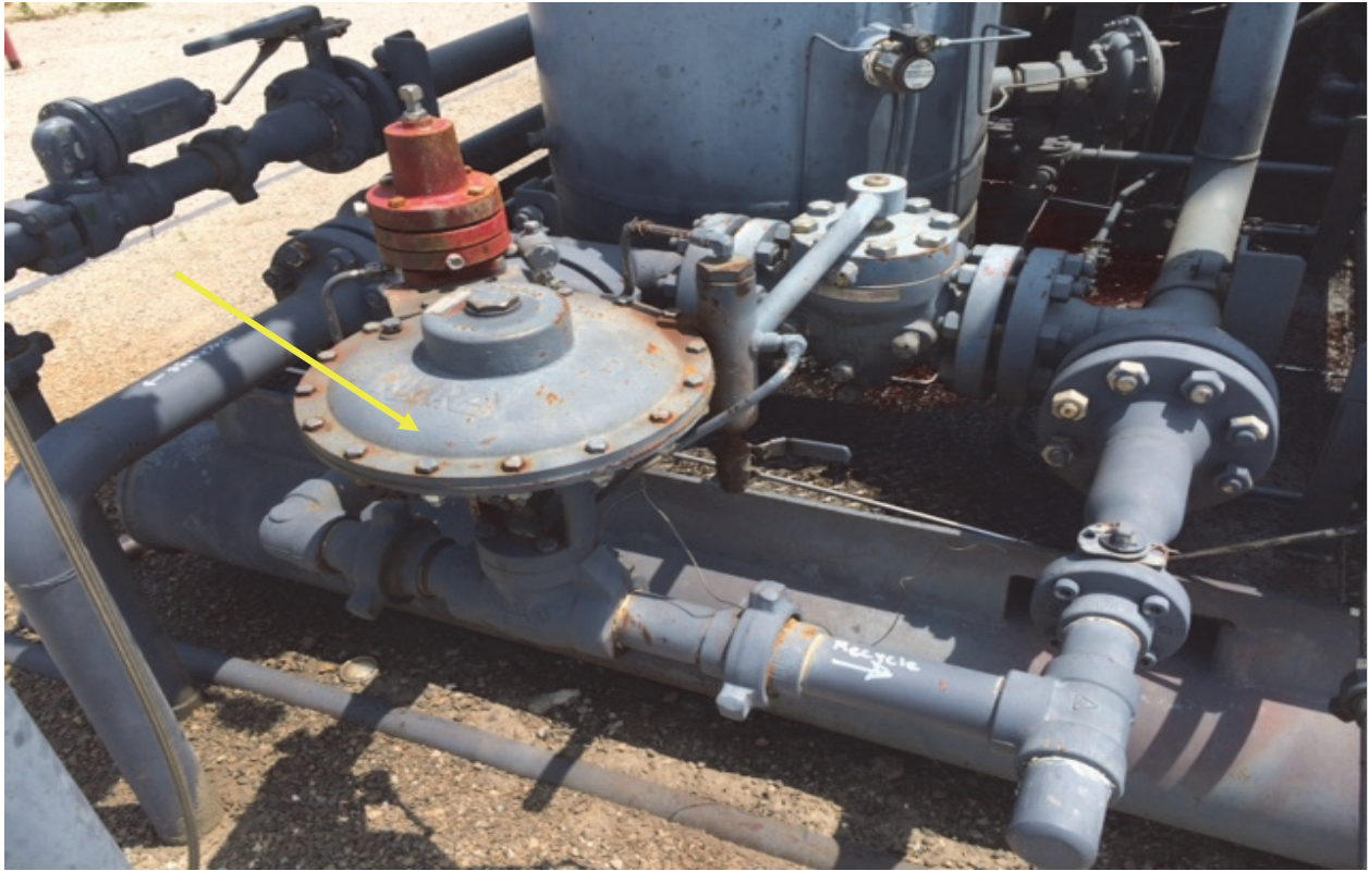
Figure 30: An on-skid recycle valve system with automated control valve, connected to the flanges of a starting bypass.
