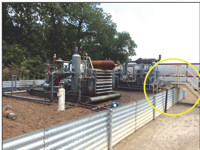
Figure 9: Locating compressors inside a containment wall inhibits truck/crane access.
