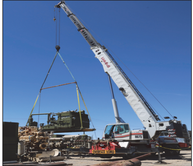
Figure 21: Smaller compressor packages can normally be moved in a single lift.
