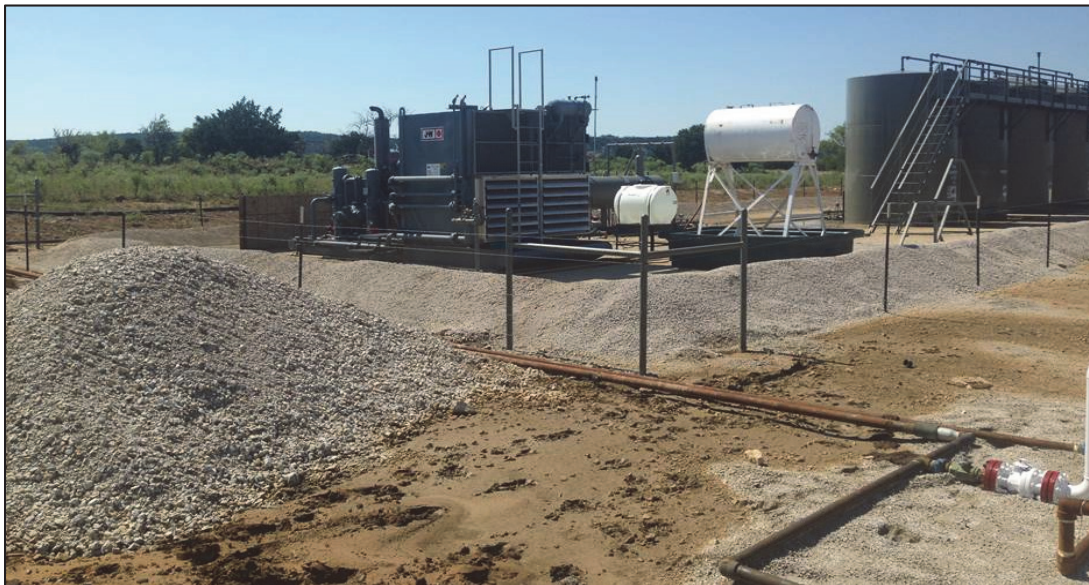
Figure 11: The location of this compressor package in the corner of a containment berm with fencing inhibits access and quick exit by operators in an emergency. The surface piping poses a trip hazard.
