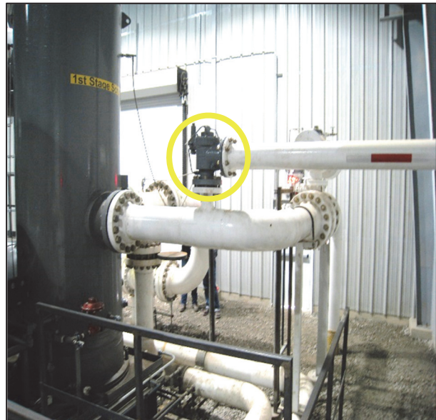
Figure 8: Pilot-operated PSV mounted on suction piping off-skid.
